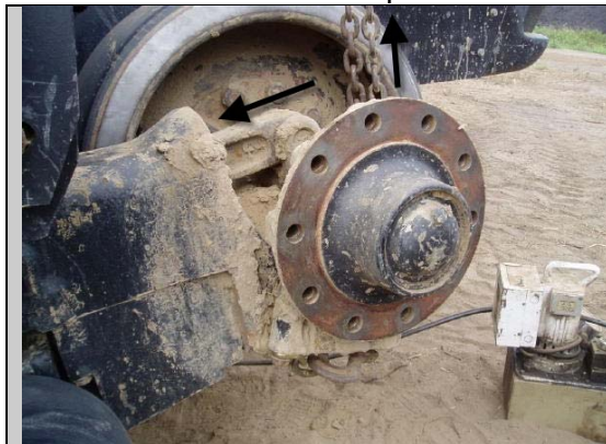
Pulling up on chain to retract tension cylinder to aid in track installation
